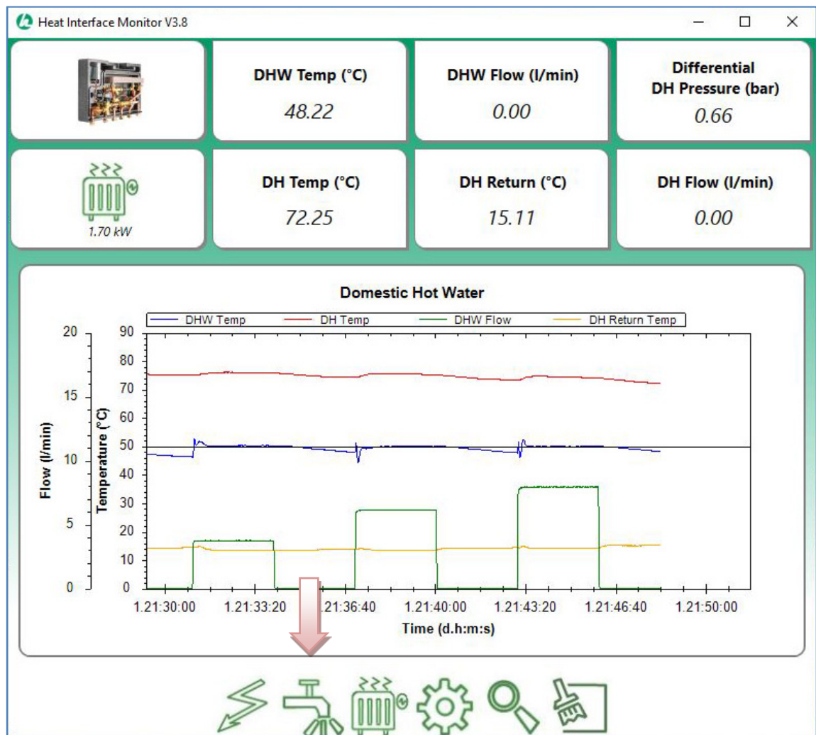
Figure 9: Domestic hot water information screen
