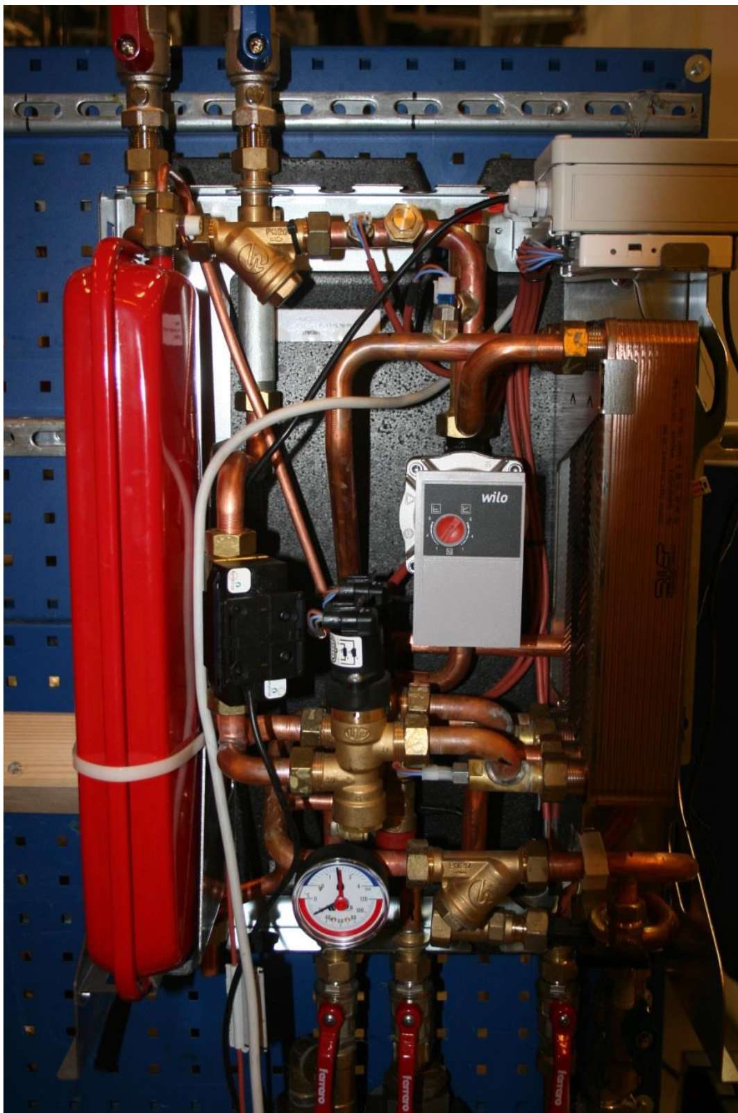
Figure 1. The test object after testing. Insulation removed.
