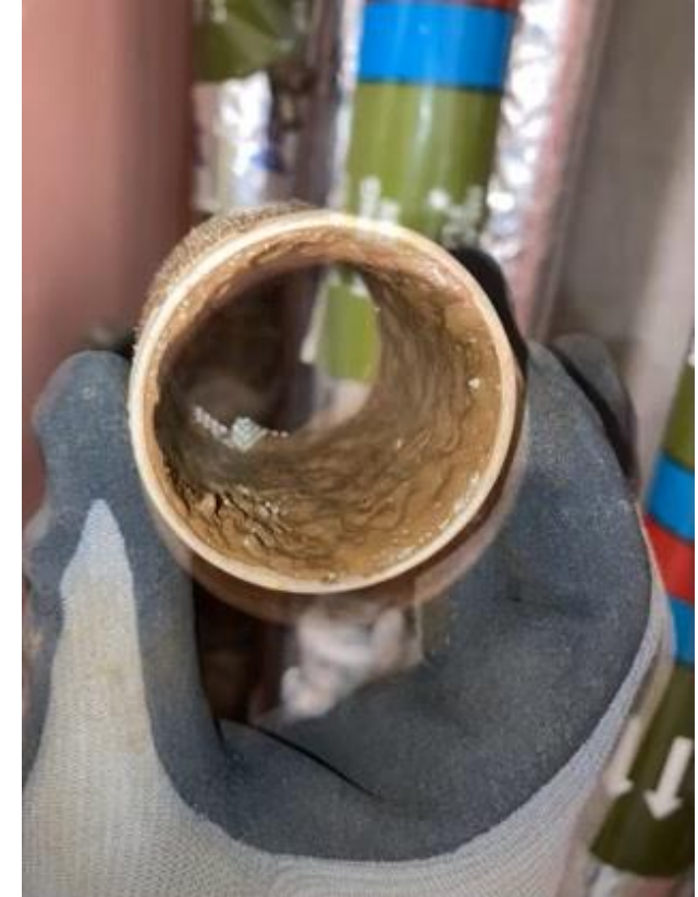
Poor water quality causes corrosion
